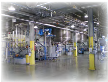
Piping to 13 Reactors for Blending Process
