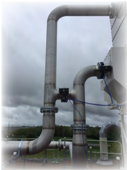
12" Stainless Steel from Fluid Bed to Dust Collector
